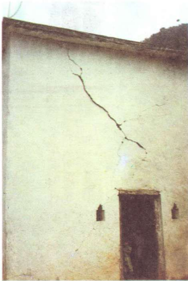
Fig. 6 Damaged house at Asena
