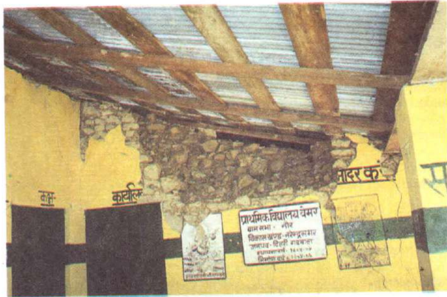
Fig. 2 Damaged primary school at Bemar
