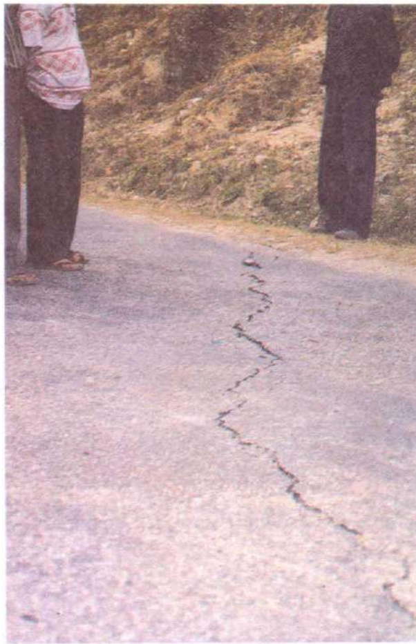
Fig. 14 Ground fissures at Indranagar
