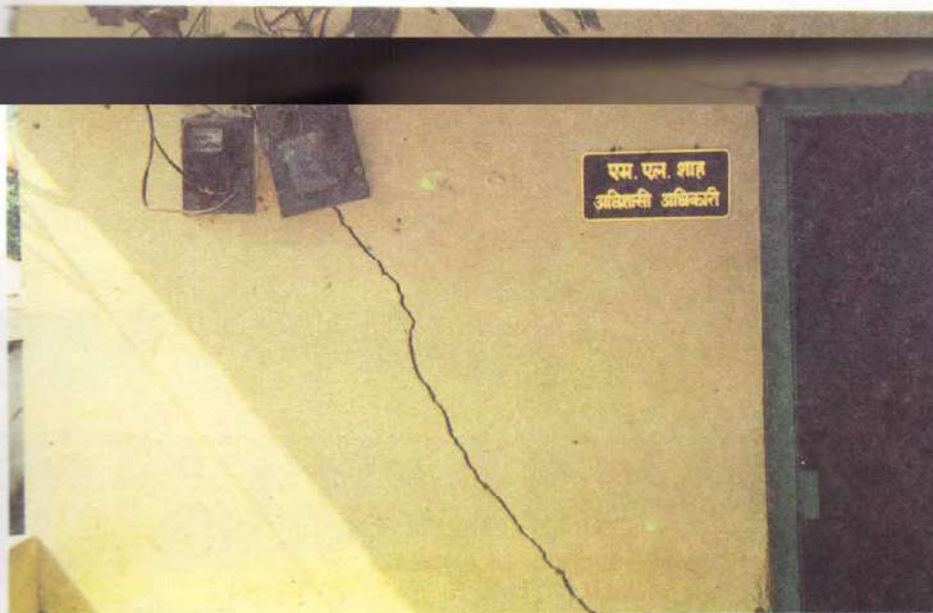
Fig. 5 Damaged house in Old Tehri Town
