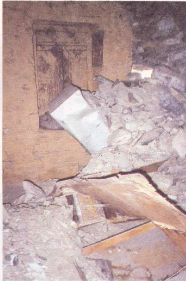
Fig. 20 Damaged house in Birhi
