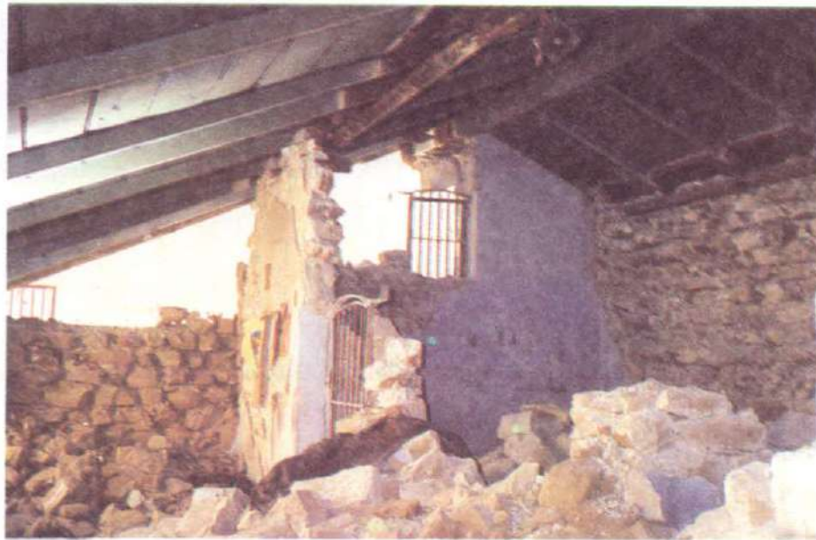
Fig. 18 Damaged jail in upper Chamoli
