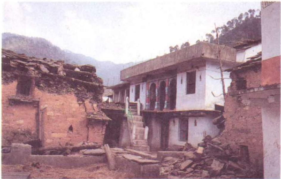
Fig. 11 Damaged house at Bhatwari Chaura
