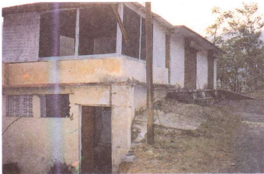
Fig. 15 Damaged house at Indranagar
