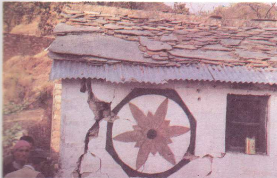
Fig.13 Damaged house at Chirbatia
