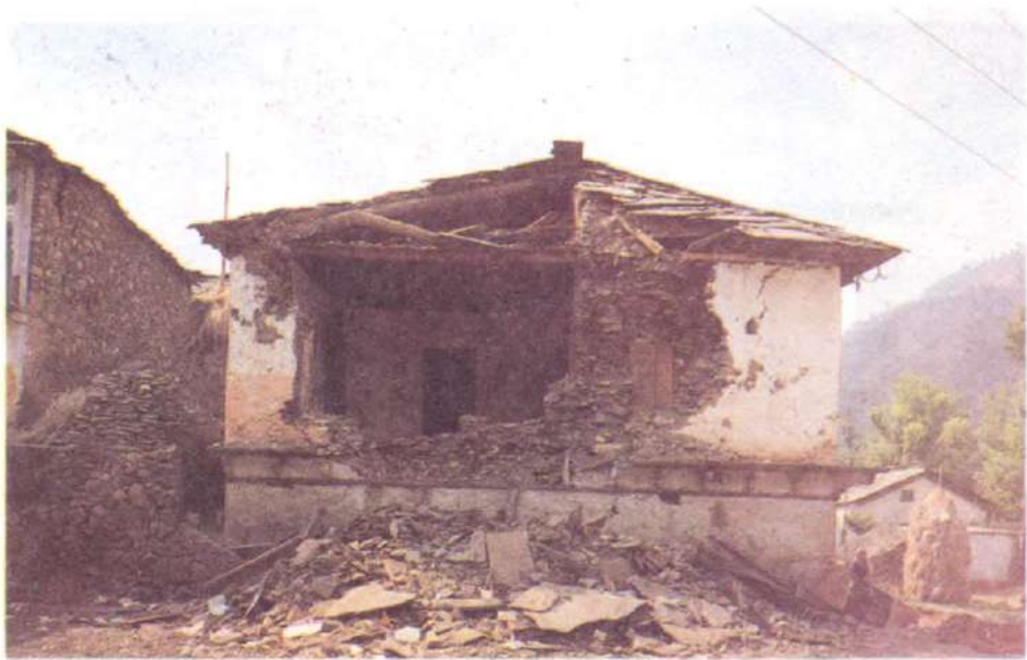
Fig. 10 Damaged house at Bhatwari Chaura
