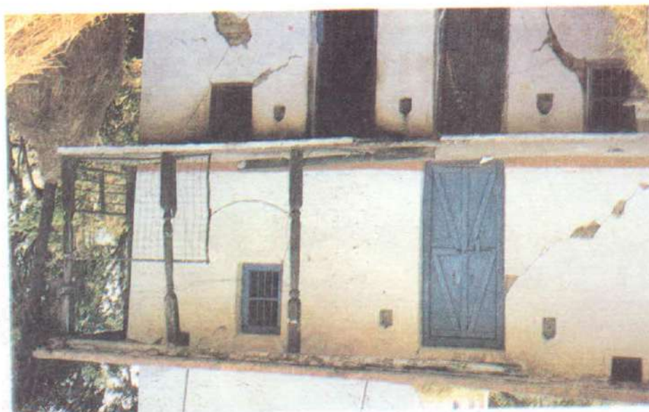
Fig. 23 Damaged house in Bhatwari Sonar
