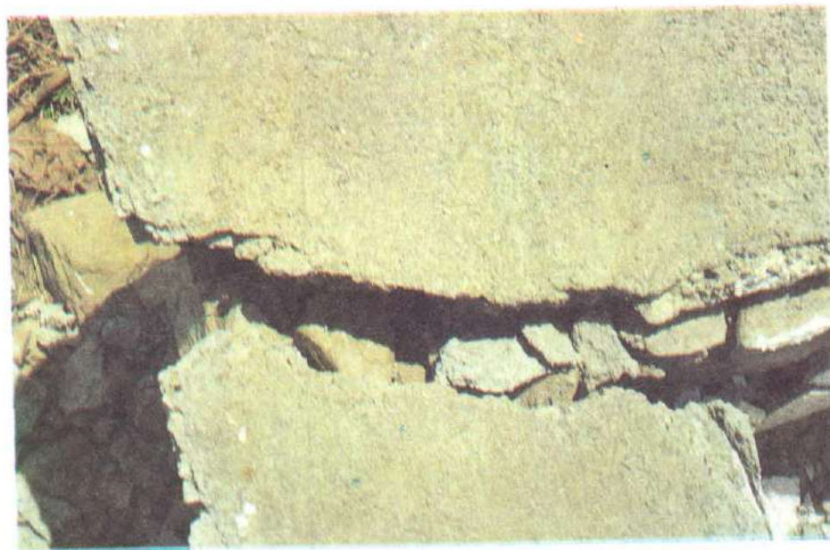
Fig. 3 Separation of boundary wall of primary school at Bemar
