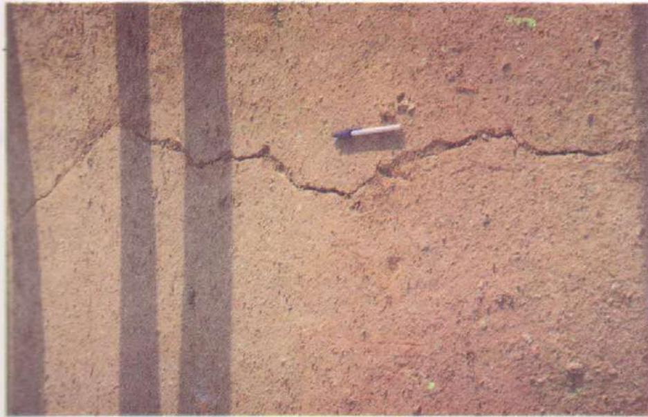
Fig. 12 Ground fissures at Chirbatia
