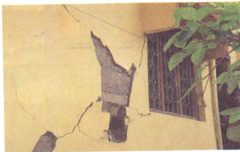
Fig. 22 Damaged house in Bhatwari Sonar
