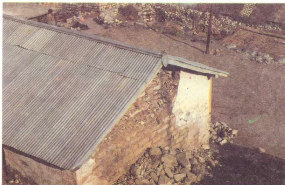
Fig. 19 Damaged house in Ghingrana
