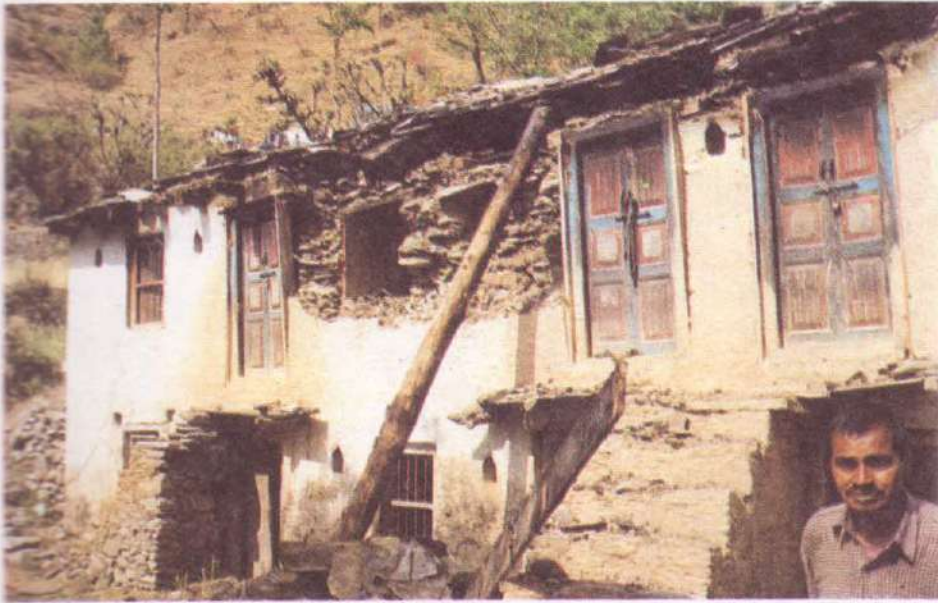
Fig. 8 Damaged house at Mehar
