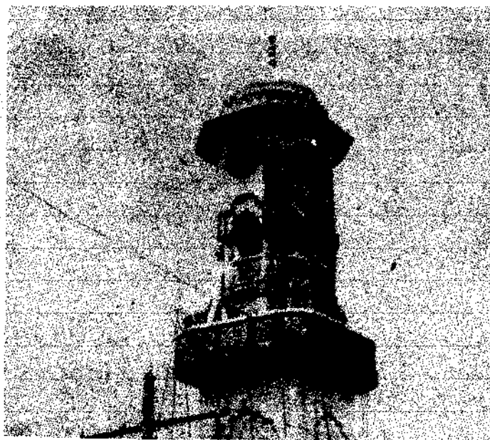
Photo 23(a) Jama masjid, Darbhanga (top portion sheared, shifted to left)
